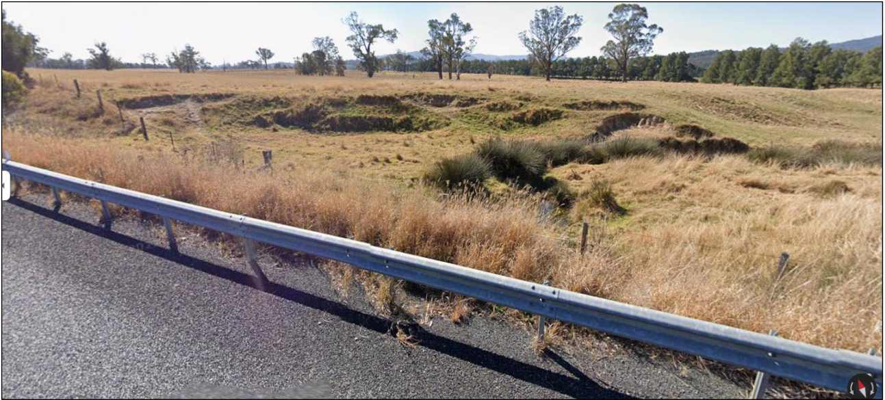
Figure 10: Looking north-east from the culvert crossing on Gresford Road. Significant erosion downstream of the culvert (image from Google Maps street view dated Aug 2023)
